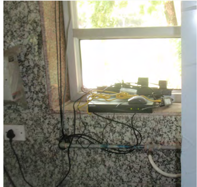
The NVR unit installed in the water cooler room from where cables approximately 20-26 feet in length connect to the two cameras outside. © A J Urfi.
