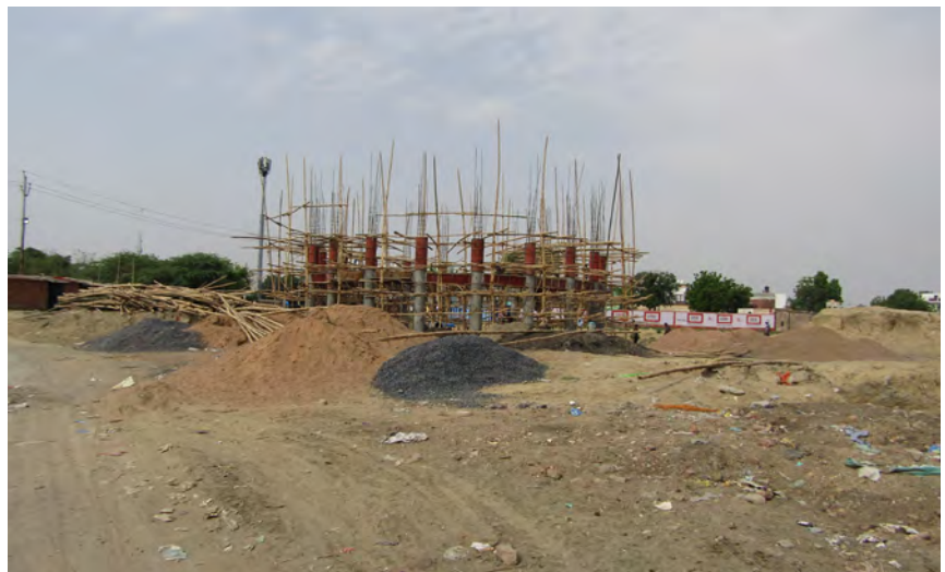
An overhead tank being constructed at the study site. © Mirza Altaf Baig.
